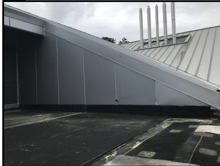
4 Asbestos results were negative for the flashing material covered by the metal panels.
